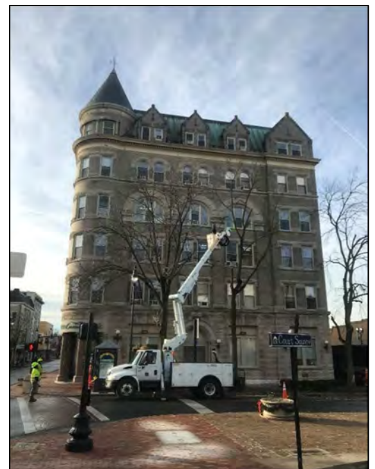
Photo 3: Ash removals at the Court Square Bank building.
