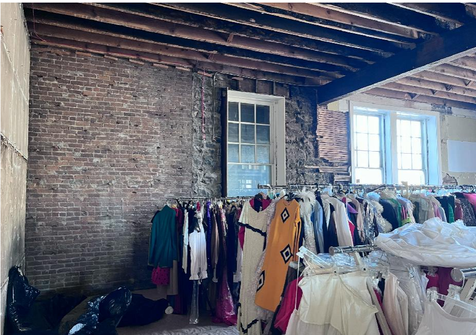
1908 BUILDING - CEILING FIRE DAMAGE
