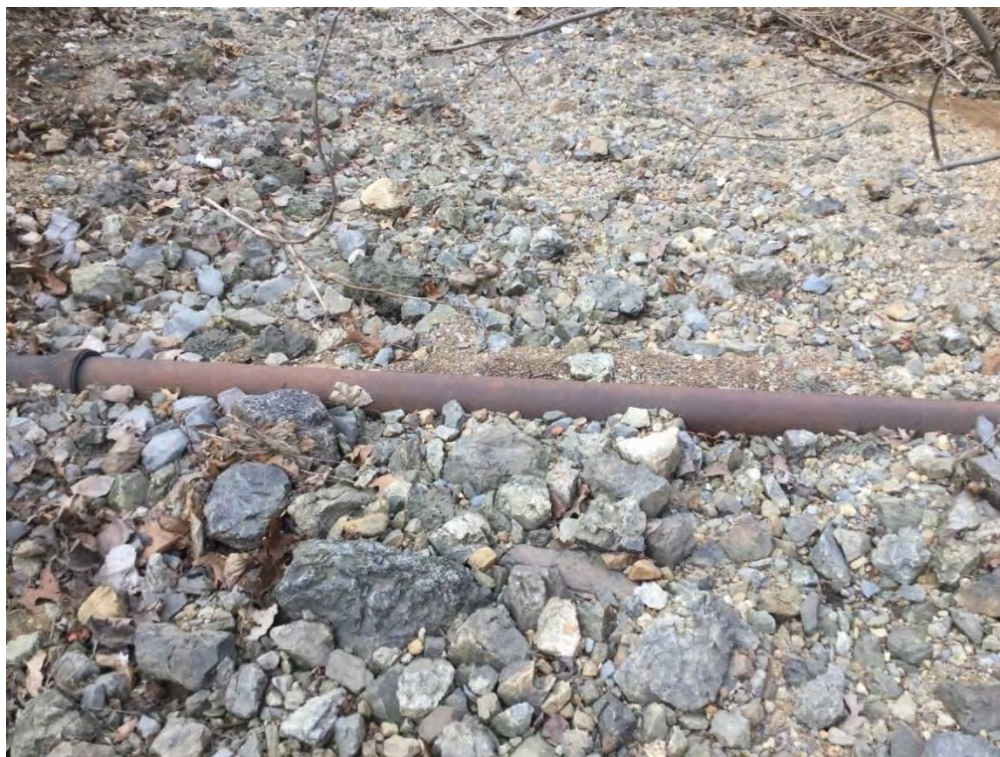
Figure 3-9 Exposed pipe in Reach 2 (6+75)
