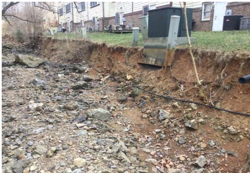
Figure 3-11 Looking upstream at eroding banks and exposed utilities along Reach 2 (7+50)
