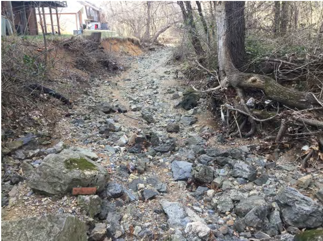
Figure 3-12 Looking downstream to eroded bank and large rocks within channel (10+00)
