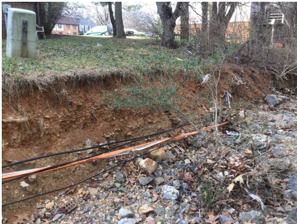
Figure 3-13 Exposed utilities along eroding bank (8+00)
