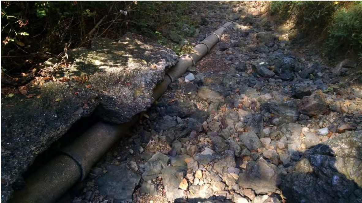
Figure 3-8 Exposed sewer line through stream section (6+00)
