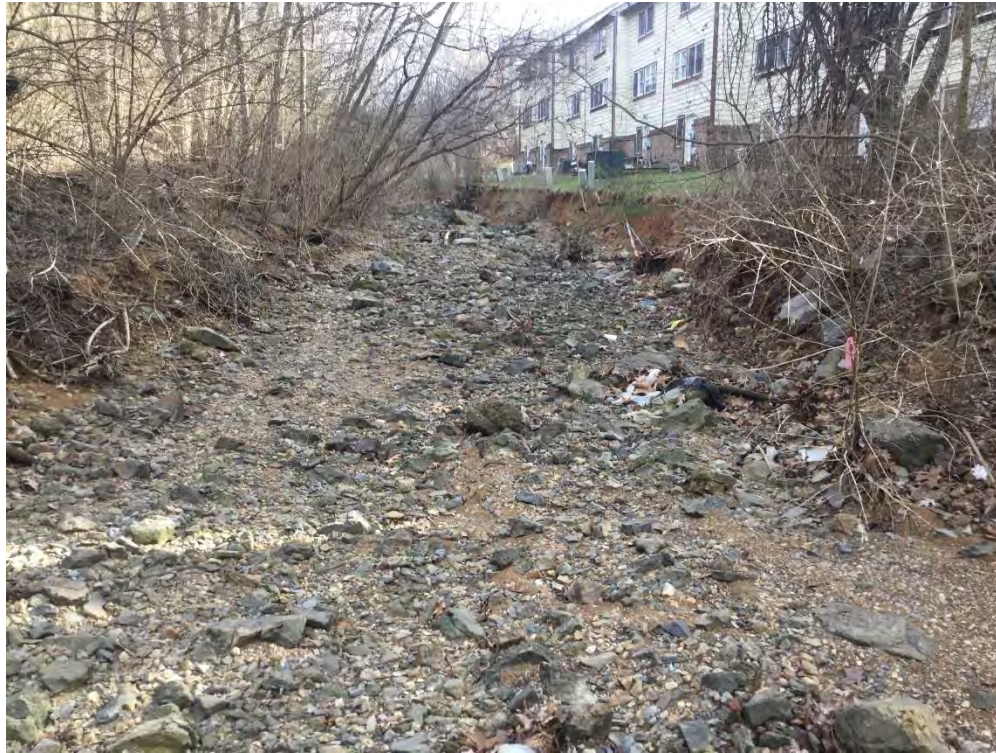
Figure 3-10 Looking up stream at eroding channel along Reach 2 (8+00)
