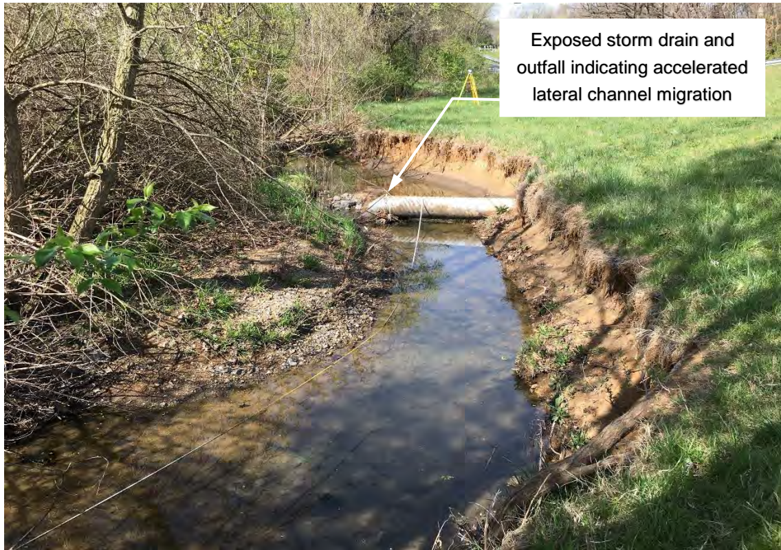
Figure 3-4 Eroded Streambank Meander Bend/exposed CMP Along Reach 1
