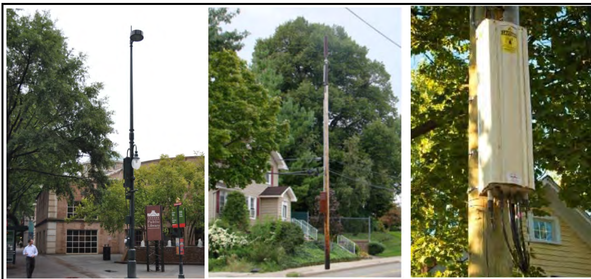
Figure 14: A DAS node attached to a street light in North Carolina 44 (left), a node attached to a wooden power pole in New Jersey 44 (center), and a close-up view of node equipment (right) 33 .
