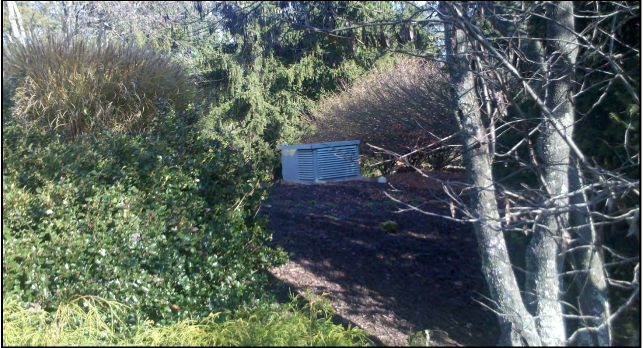
Figure 4: Rear view of the base of the concealed telecommunications flagpole. The underground equipment vault is located under this area with only the visible small piece of equipment at the surface. 26
