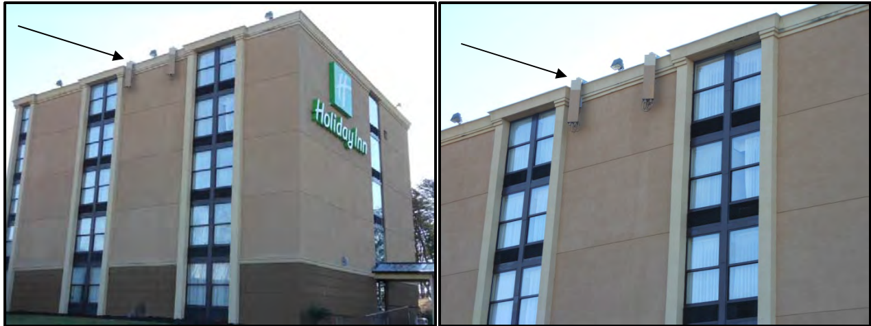
Figure 8: Flush mounted antennas painted the same color as the supporting structure at 1400 East Market Street, Harrisonburg, Virginia.
